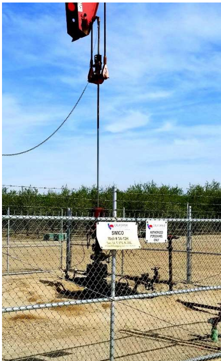
Figure 6 Well head SWICO #34-12H
